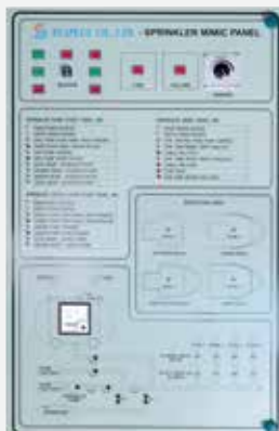
Sprinkler MIMIC Panel
