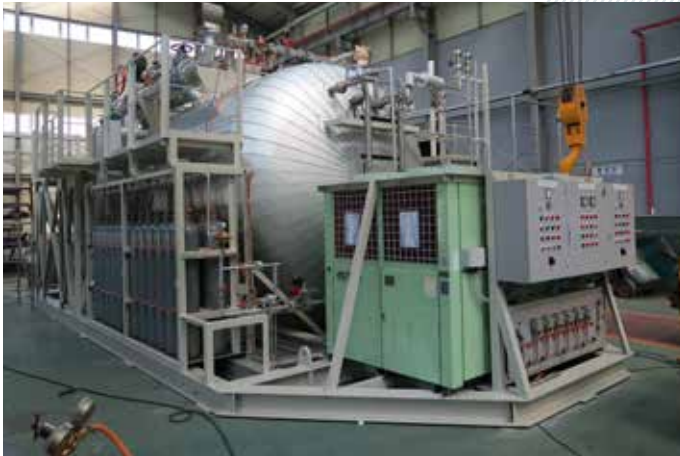
Low Pressure CO 2 Storage Unit
