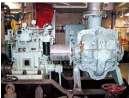
Fire Pump Unit
