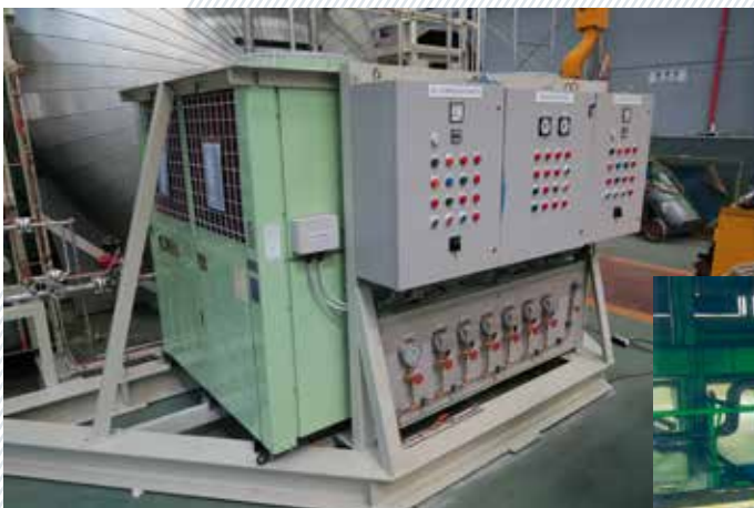
Refrigerating unit & Control Panel
